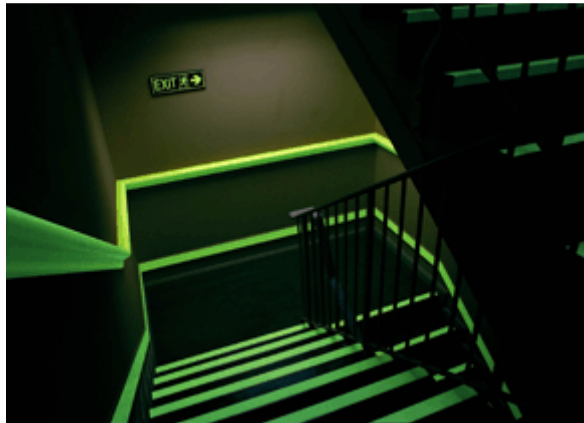
Photo: Courtesy of Jalite Group IBC 2009 requires the use of luminous egress path markings in various occupancy groups with special provisions.
